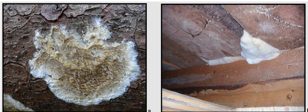
Fig. 2. Example of erosion of an oak beam caused by fungi: a. The initial stage of development of the Coniophora Puteana fungus on a cut tree beam; b. Initial stage of development of Serpula lacrymans fungus on wood.
