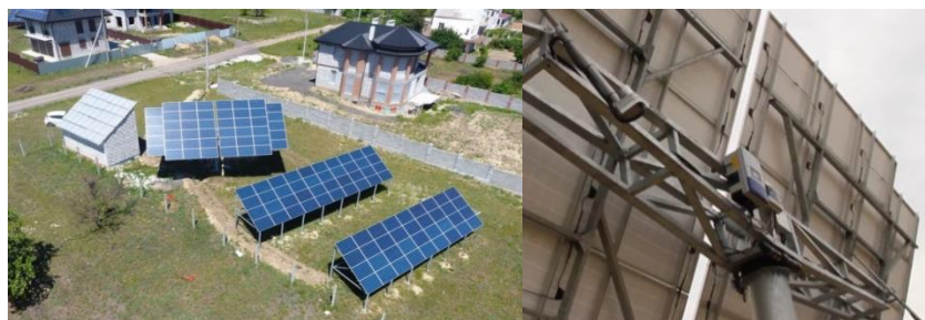
Fig. 2. General view of mounted solar trackers.
