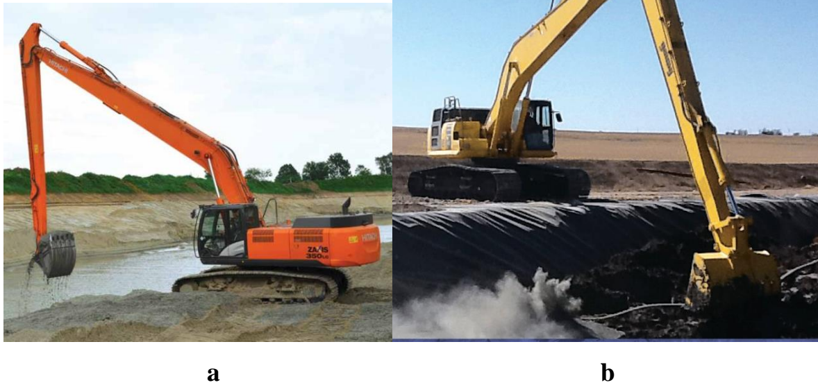
Fig. 3. Excavators with increased digging reach during operation: a) Hitachi ZX 250LC clearing a channel; b) Komatsu PC 240LC-10
