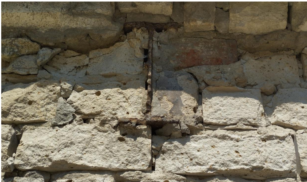
Figure 2. Surface and structural damage to wall material
