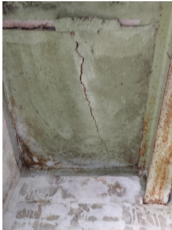
Figure 3. Structural cracks in the monolithic covering of the outbuilding
